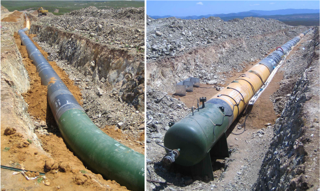
Figure 2 – X100 line A (on the left) and line B (on the right) fully instrumented.
