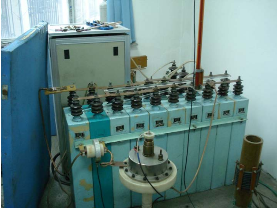
Fig. 3.1: Capacitor bank and its charging setup
